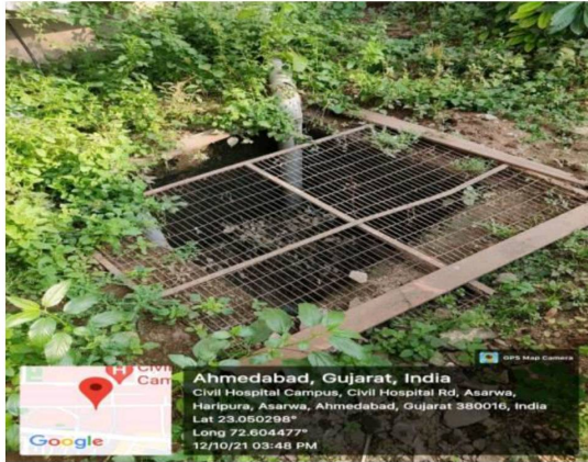
Rain water harvesting system
