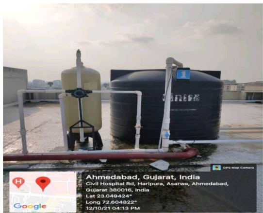
Water distributing system
